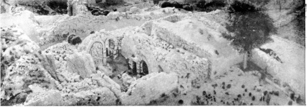
Fig. 1. A house in Nebi Şamwîl in process of building. It shows the crescent-shaped walls, ready to be vaulted.
